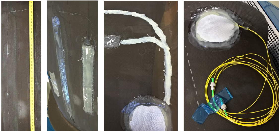
Fig. 6: FBG sensor installation procedure (from left to right): 1. Optical fibre fixed on the air intake surface; 2. Covering layer applied over the FBG sensors area (thin Glass fabric / Epoxy resin); 3. Covering layer to protect optical fibre routing (mixture of epoxy resin and micro-balloons); 4. Glass fabric protection of fusion splices and optical pigtailed with FC/APC connectors
