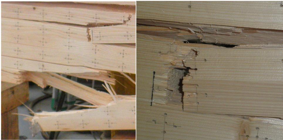
Fig. 2: Destruction of the finger joint
