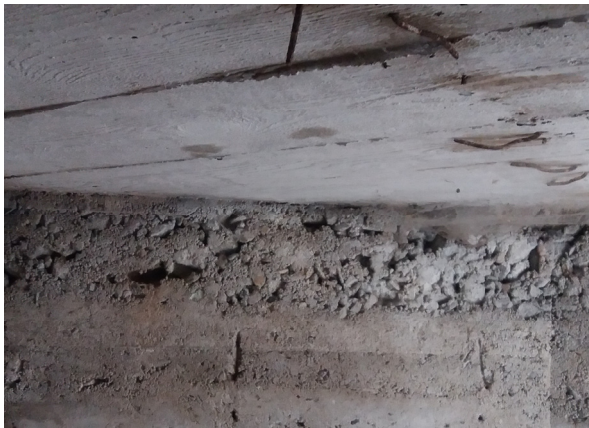
Fig. 3: Different quality of concrete.
