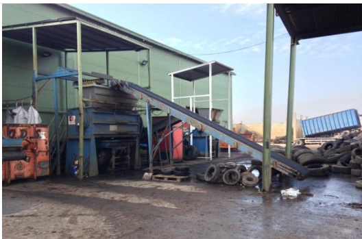
Fig. 1: General view of the shredding machine with a conveyor
