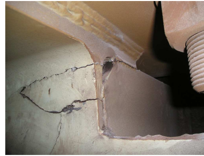
Figure 4: Cracks in the pedestal of the converter's torsion system in the location of the weld between the vertical console and the flange as well as in the I-beam's web.
